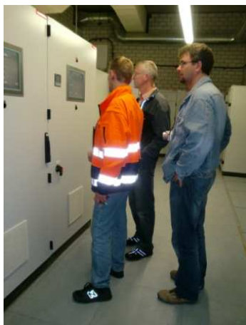
Complex infrastructure in the tunnel
