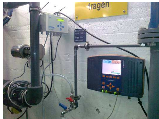
Display and documentation with a “Disinfection Controller” from ProMaqua
