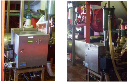
Picture 4: OilGuard installation on an oil platform
