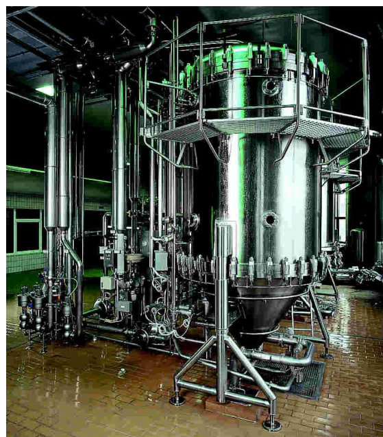
Picture 2: Typical Kieselguhr filtration plant
