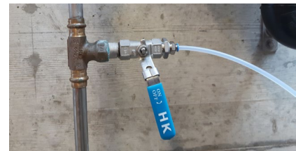
Figure 5: Simple control of the required water flow rate of 200 to 400 ml/min when continuously measuring with the BactoSense
